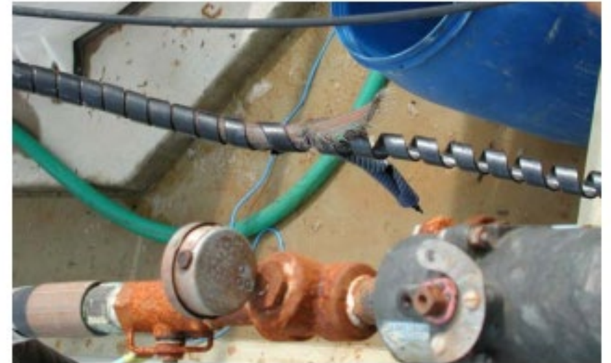
Figure 2. Failed stainless-steel transfer hose.
