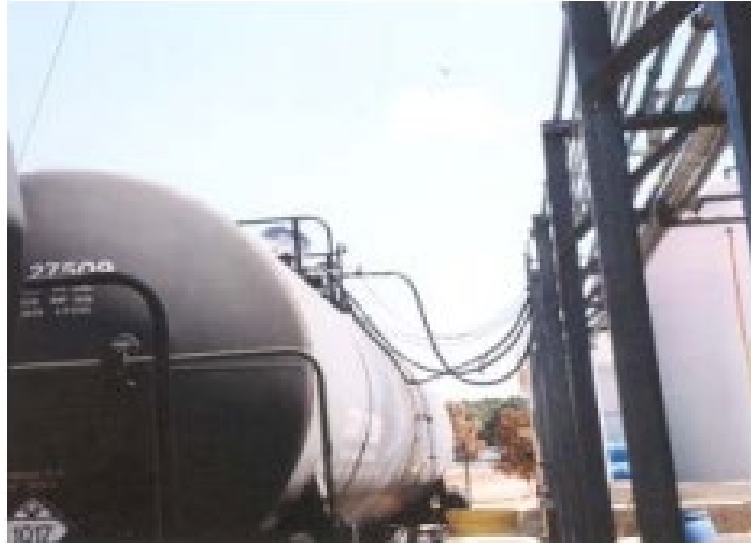
Figure 1. Railroad tank car unloading station #3.
